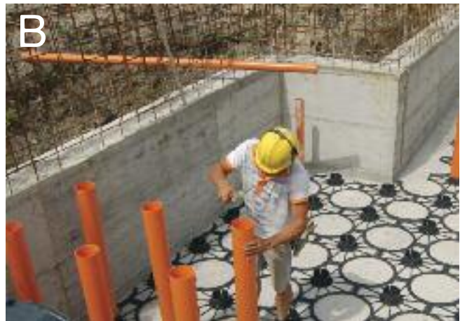
Fig B. The concrete slab and walls should be constructed to Engineer's specification, and the formwork installed.
