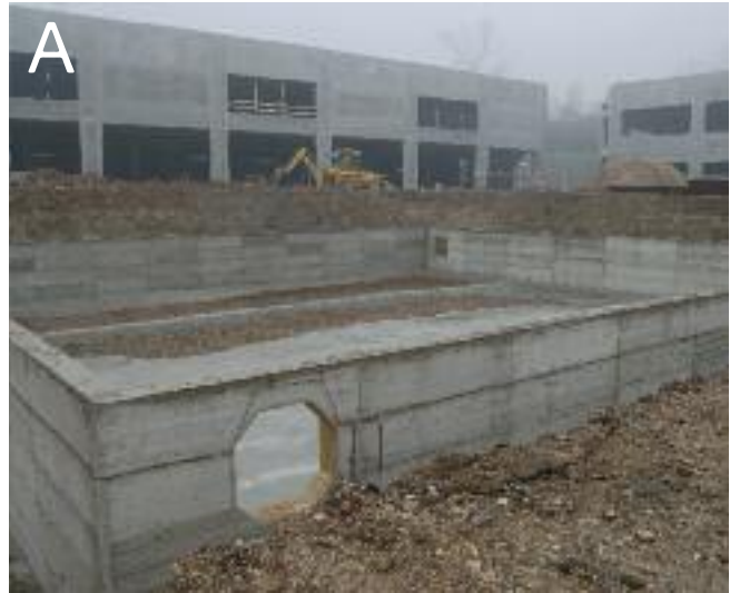
Fig A. The ground should be excavated to the required depth including the battering of sides to ensure stability, then the area should be filled with compacted gravel.
