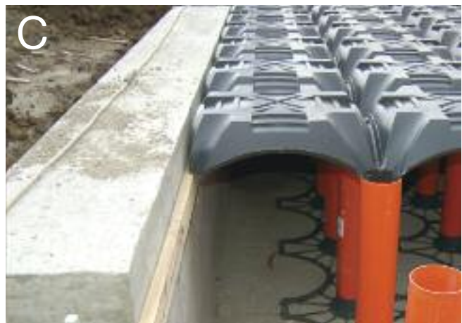
Fig C. Ensure the outside edge of the first row of forms rests securely on the pre-fixed batten
