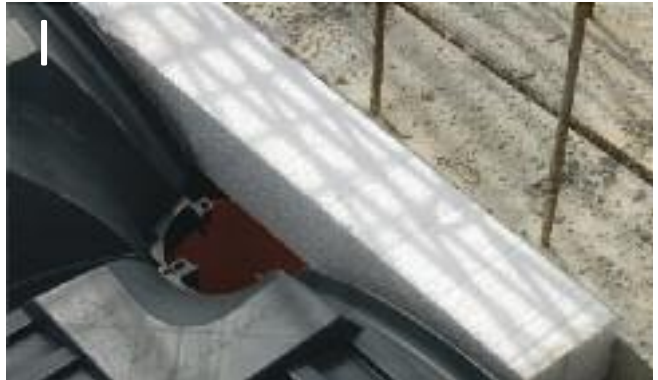
Fig I. A polystyrene fillet piece placed between the tank wall and the first row of forms, to fill the gap when the first row of columns is close to the wall.
