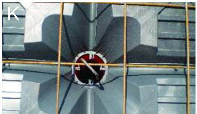
Fig K. U-bar reinforcement is placed inside every column, hung over the bars of the welded wire mesh. Ensure that the bars are long enough to reach the bottom of the columns.
