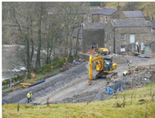
Banbridge Hydro Scheme
